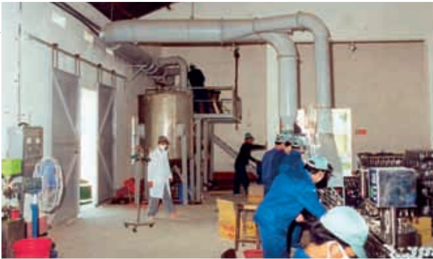
The collection system for toxic substances, installed in a pesticide-manufacturing plant.
